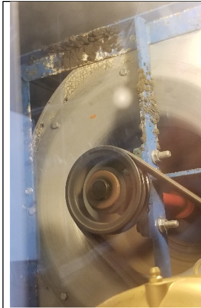
Fan Section – Mold Contaminated
