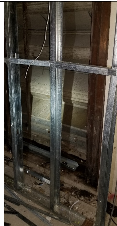
Existing AHU air intakes pulling from the new construction area.
