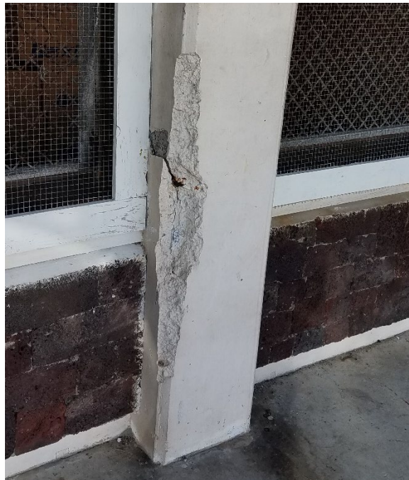
Figure 5: Concrete spalling at bent, typical.
