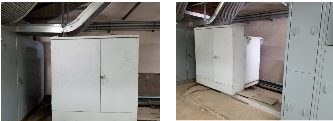
Old Main Transformer and Old Service Transfer Board, with New Generator Switchboard Behind
