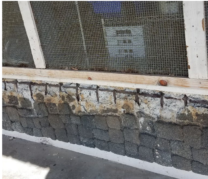
Figure 6: Concrete spalling at kitchen stem wall.
