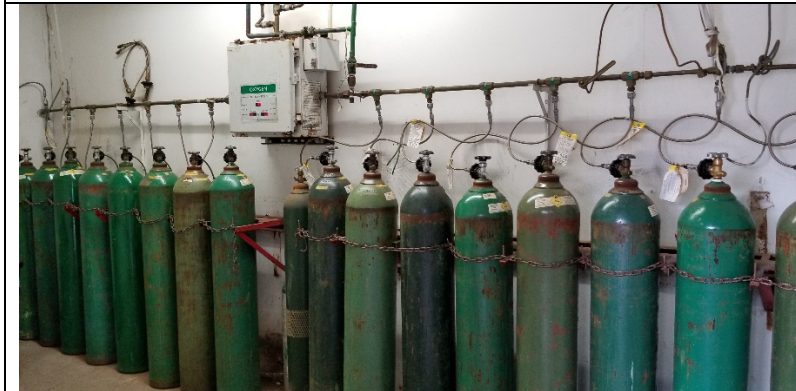
Non-Functional Oxygen Manifold
