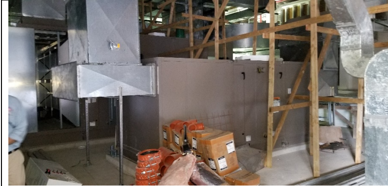
New Air Handling Units.
