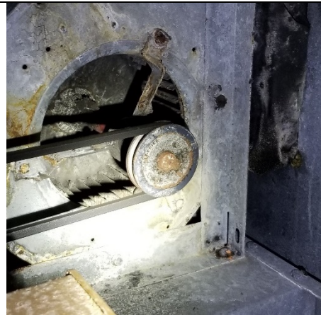
Air handling unit – fan not functional
