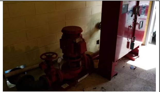
Fire Water Booster Pump
