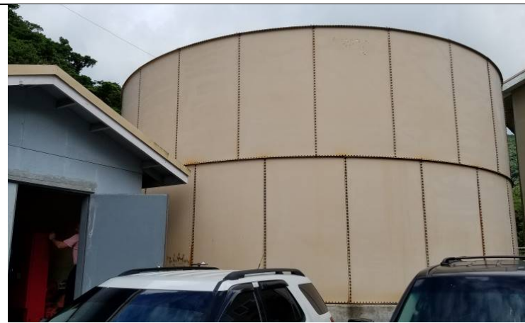
120,000 gallon Domestic and Fire Water Storage
