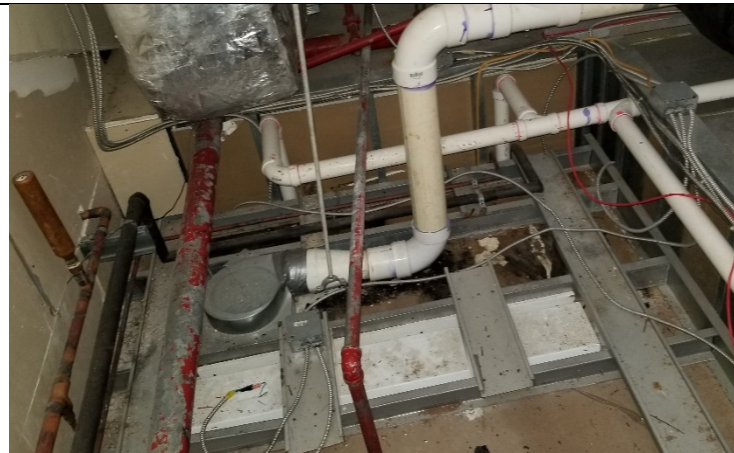
View of the ceiling from the mechanical mezzanine - no rated partition or barrier
