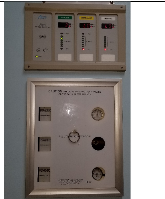
Typical Zone Valves and Area Alarms in Patient Wards
