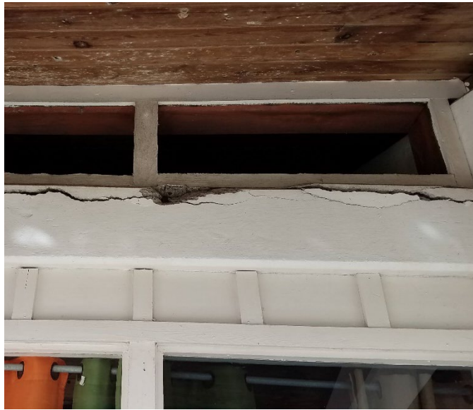
Figure 4: Concrete spalling at bent tie beam, typical.
