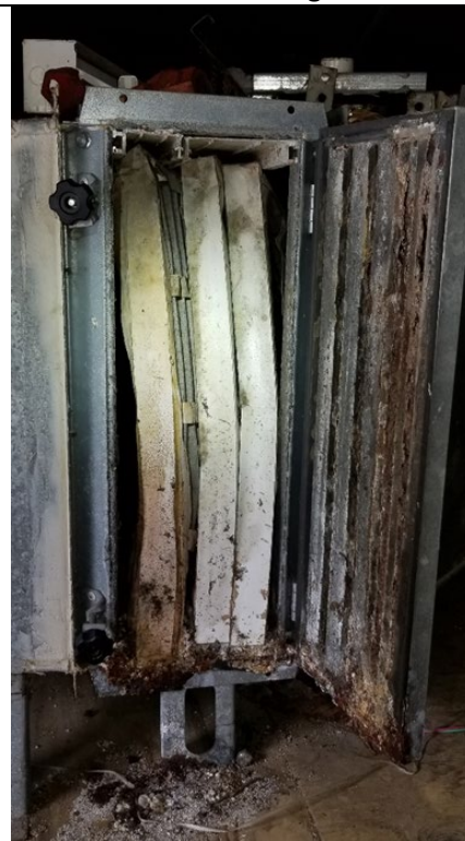
Outside Air Filters
