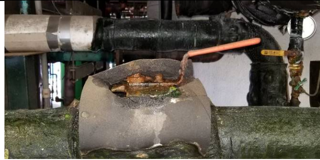
Primary Chilled Water Piping
