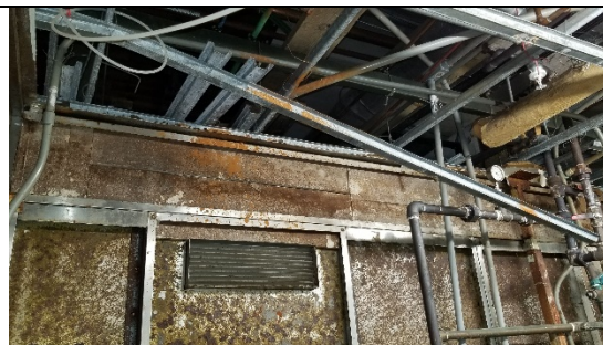
Sterilizer equipment room open to unconditioned ceiling plenum
