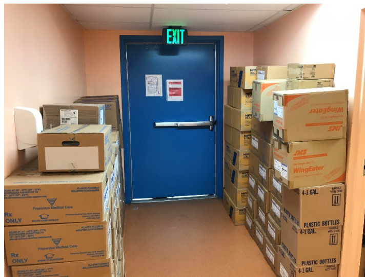
Rear of Dialysis Clinic with Combustible Storage in Corridor
