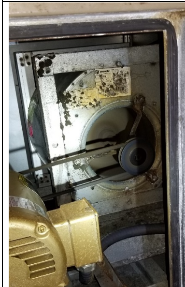
Typical Fan Section – Mold present
