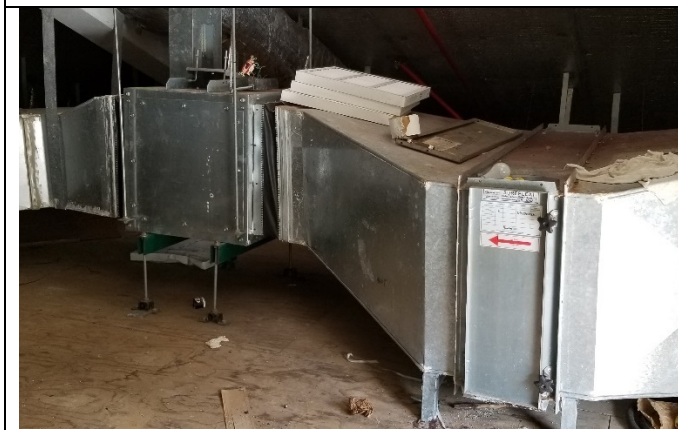
Outside air supply fan (motor missing).
