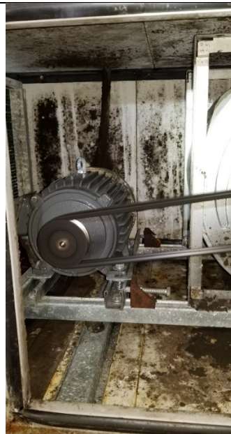
Air handling unit - fan section - mold present
