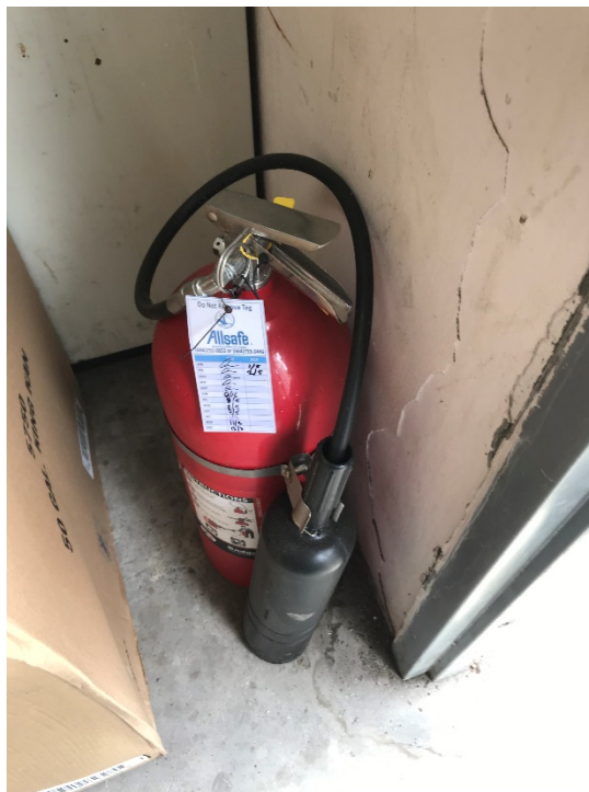
Unsecured extinguisher in central plant, not inspected on a 30-day cycle.
