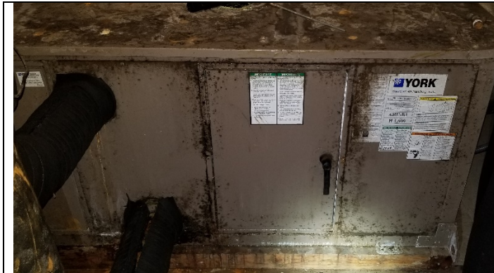
Typical air handling unit (Medical Ward) – mold present
