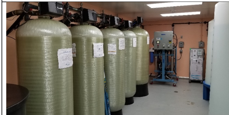
Dialysis Water Treatment
