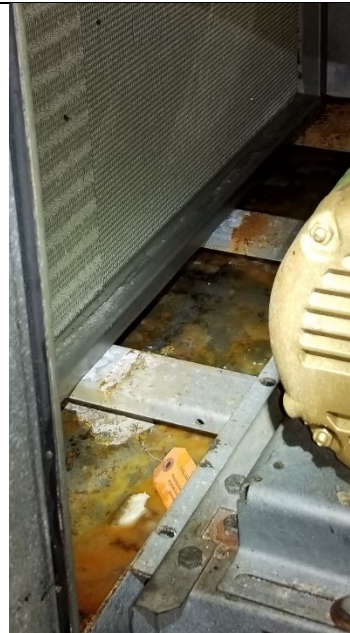
Typical Cooling Coil Drain Pan – mold/biofilm present
