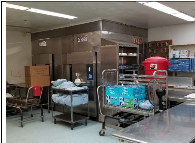
Sterilizer – Loading / Unloading
