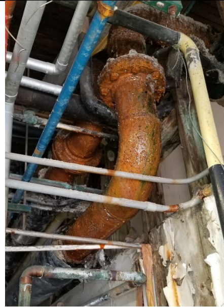
Secondary Chilled Water Piping
