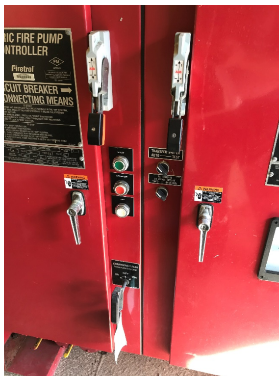
Fire Pumps with Breaker Disconnected
