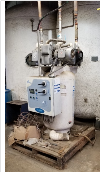
Medical Vacuum Pump (operational)
