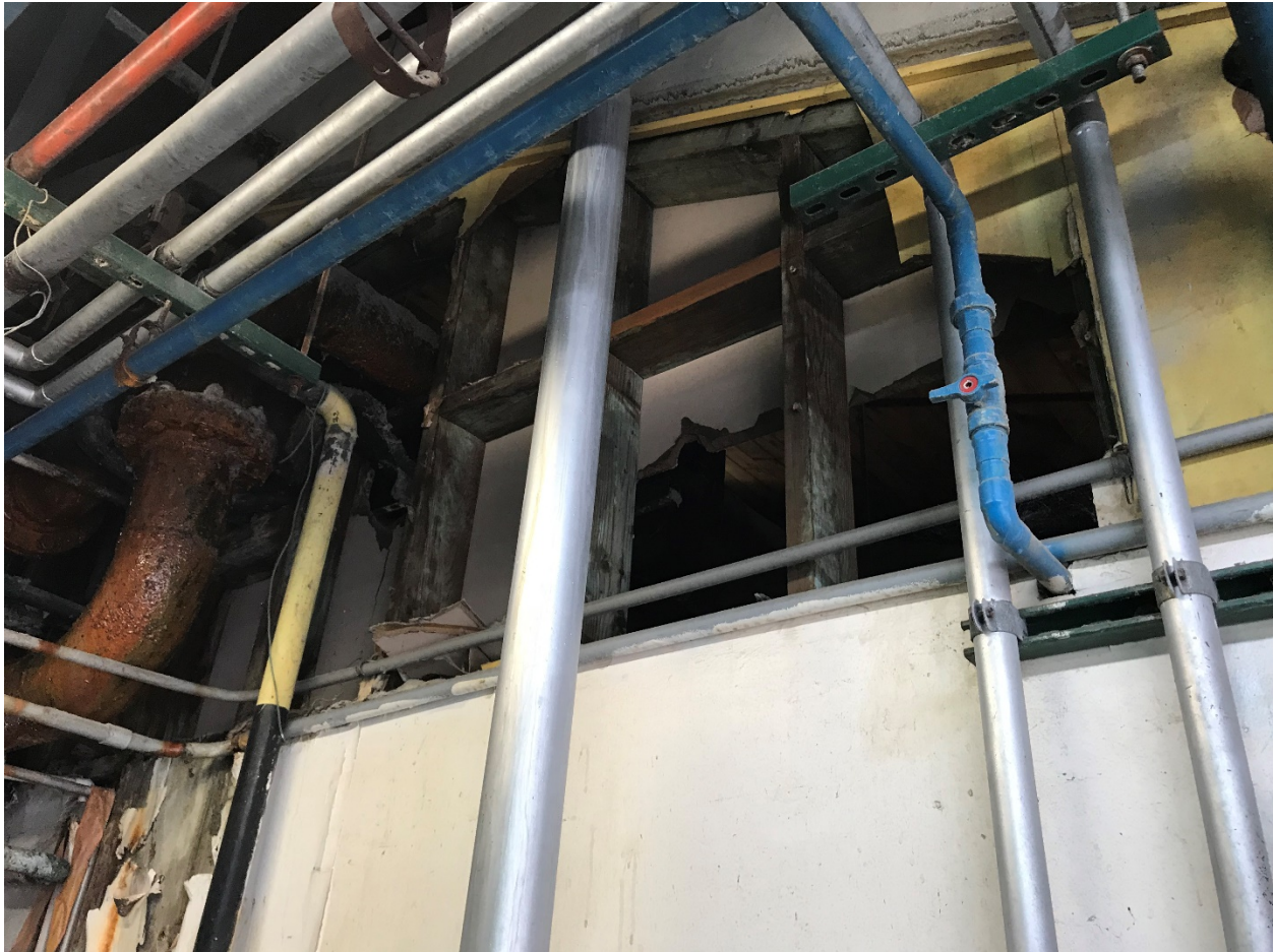
Lack of Firewall Separation in Central Utility Plant
