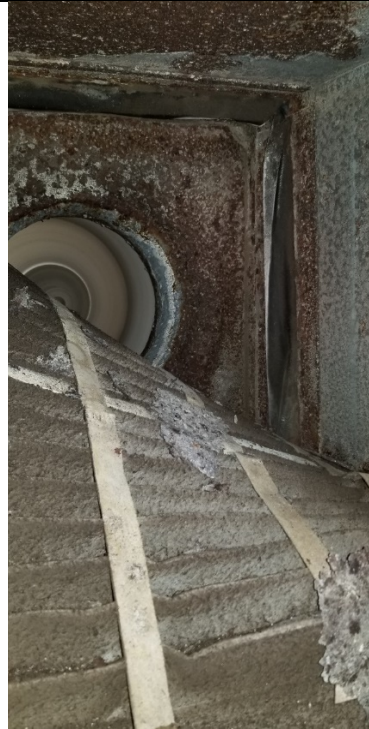
Outside air fan and filter
