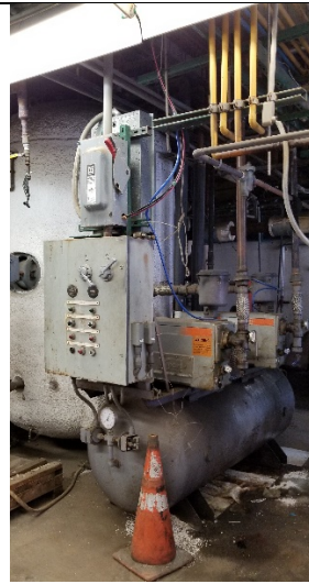
Old Medical Vacuum System (abandoned)
