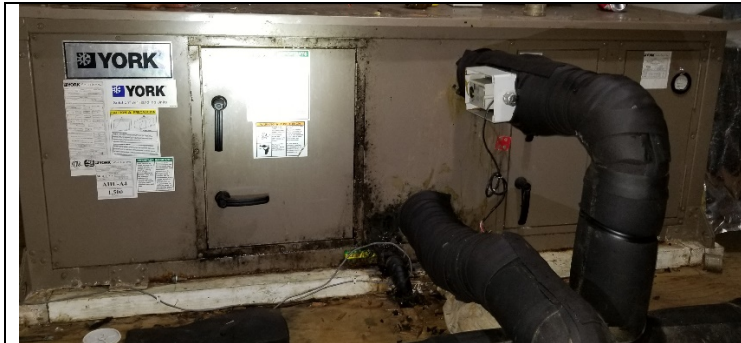
Typical Recirculation Air Handling Unit (Pediatrics Ward)
