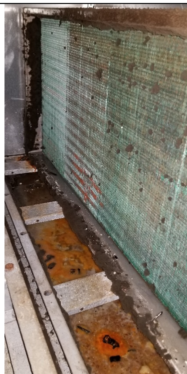
Typical cooling coil and drain pan.
