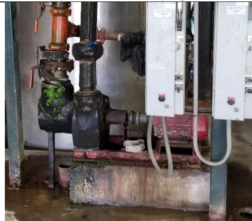
Primary Chilled Water Pump
