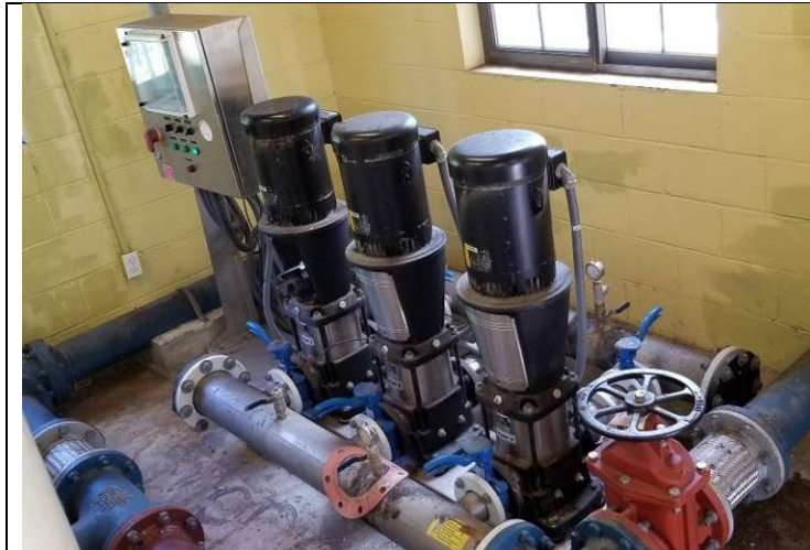
Domestic Water Booster Pumps
