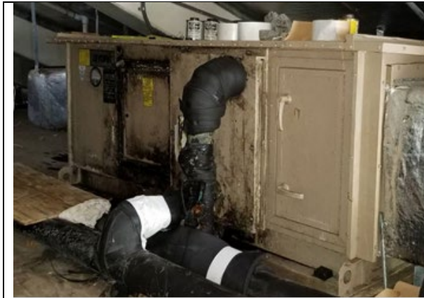
Air Handler – Surgical Ward
