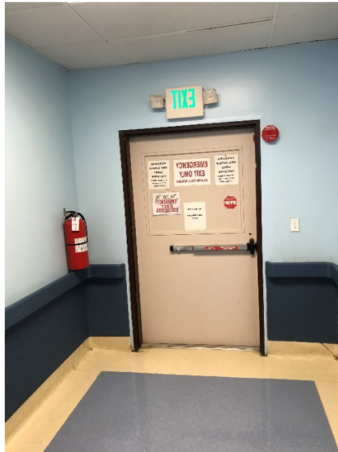
Exit Door from the Surgical Inpatient Ward in compliance with NFPA 101
