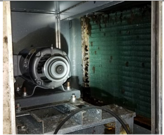
Fan Section and Cooling Coil
