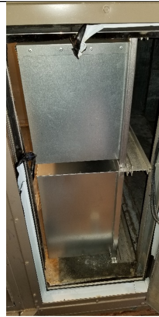
Air Filters – Merv 11 Filters installed. Prefilter frame present but no filter installed.
