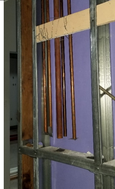
Uncapped/Unpurged Med Gas Lines
