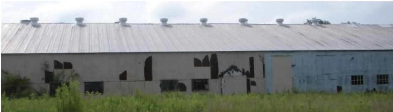
Abandoned historical building on the Crab Orchard National Wildlife Refuge near Marion, IL. These former on-site facilities have been leased to industrial and commercial tenants for re-use. (Photo: FWS)
