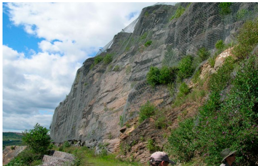
Fencing used to protect hikers from rock slides. (Photo: Greg Nottingham, NPS)
