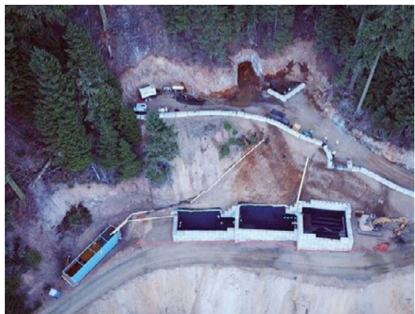
Bulkhead installation in progress at the Formosa Mine Superfund Site. Temporary water treatment system installed during the bulkhead replacement project. (Photo: John Barber, BLM)
