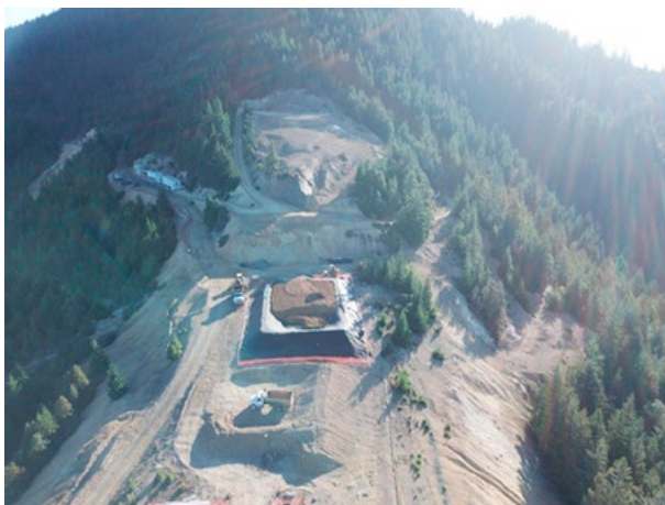
Temporary mine waste repositories being constructed at the site during bulkhead installation. (Photo: John Barber, BLM)
