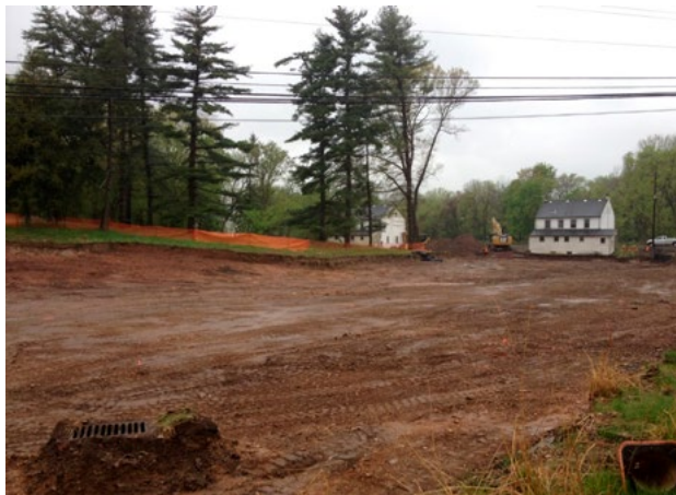
Before: Soil excavation and remediation activity at the Valley Forge NHP. (Photo: NPS)
