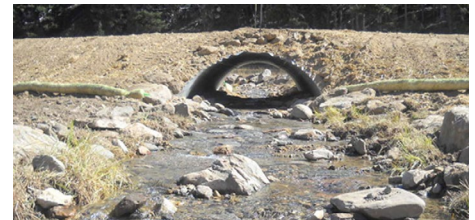
Small creeks with inadequate fish passage habitat and connectivity can increase flood risk, decrease the resilience of aquatic species, and contribute to the loss of self-sustaining species. This set of photos show the conditions before (top) and after (bottom) restoration work at a small roadway creek crossing. Photo credit: USFWS
