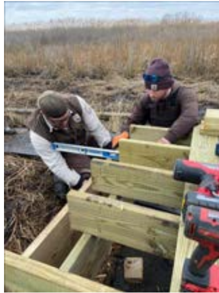
Figure 4: GAOA MAT Strikeforce Team Members Constructing a Replacement Boardwalk at Eastern Neck NWR
