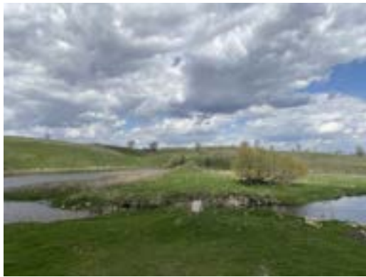
The levee and culvert before repairs.
