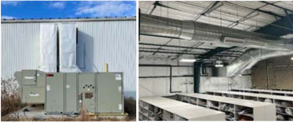
The new HVAC system outside and in the storage area of the National Eagle Repository.
