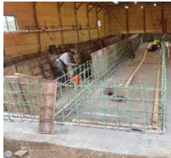
Genoa National Fish Hatchery, Wisconsin, replacing the old fiberglass indoor fish production raceways with long lasting concrete raceways. Photo credit: USFWS
