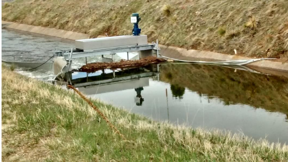
Debris clogged in the hydrokinetic generator's rotors. Tarp transitions were cut to relieve upstream water levels. Photo: Bureau of Reclamation.
