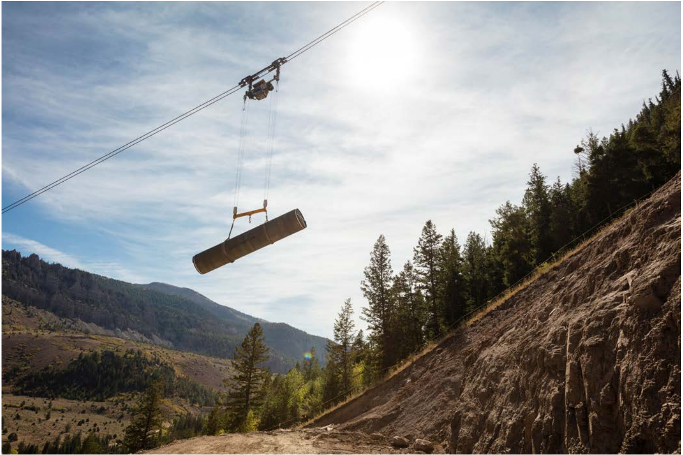
A cableway crane is used to hoist a 40-foot-long section of 84-inch-diameter welded steel pipe from the valley floor for installation on the steep canyon slope as part of the North Fork Siphon Replacement Project, Central Utah Project.
