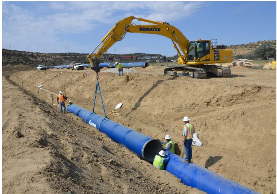
Pipeline installation on the Navajo-Gallup Water Supply Project in support of Tribal and underserved communities.
